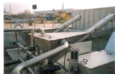
Grit & Sand Separators
