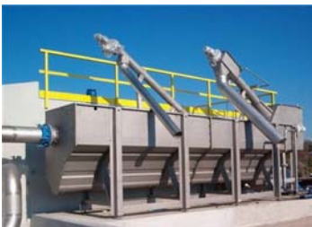
TOP Combined Systems (Screening, Grit & FOG Removal)
