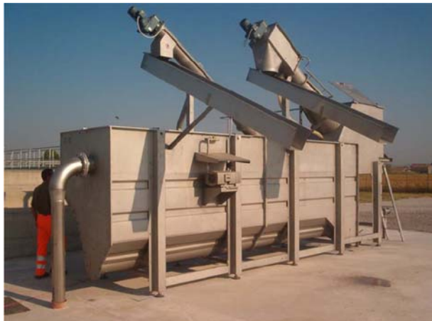
Typical TOP Combined System installed at a waste water treatment works to receive tanker imported sewage from cesspools and septic tanks.
